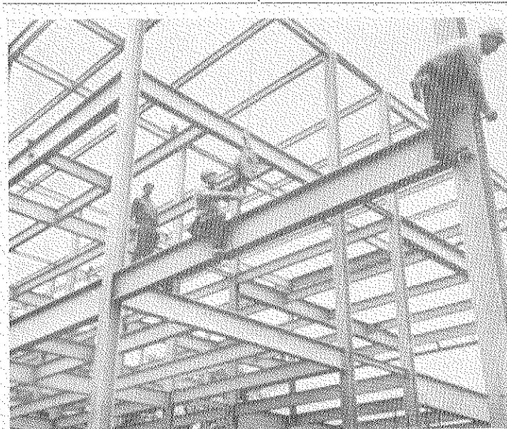
STEEL GIRDERs erected for a $1.5 million addition to the research facilities of The Goodyear Tire & Rubber Company are protected against corrosion by a material developed by the Company for the paint industry. A primer coat of paint based on a synthetic rubber resin was applied to the girders at the steel fabricating plant. A finish coat of paint made from either the rubber resin or an acrylic type resin, also developed by Goodyear for paint formulations, will be used on both exterior and interior steel surfaces.
