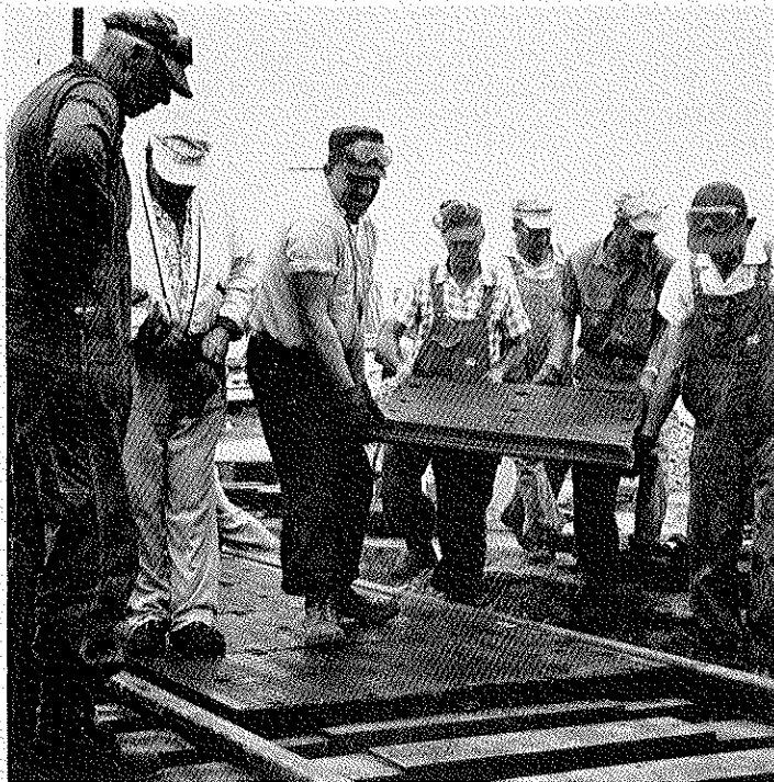
RAILROAD CROSSING PADS made of rubber bonded to steel are an exclusive Goodyear product. Their manufacture is confined to St. Marys.
