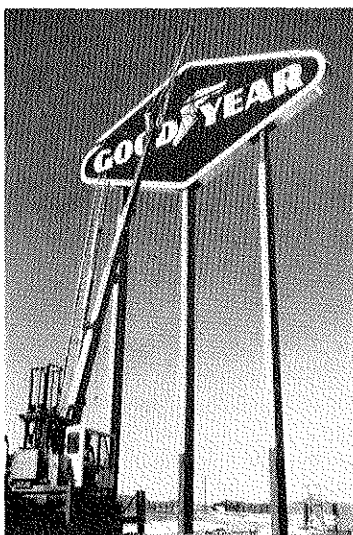
THE ERECTION of the Goodyear sign on Route 23 required a great deal of skill to "Protect Our Good Name". More construction details are shown on Page 3.
