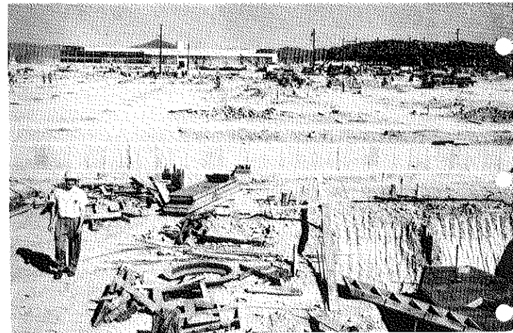
X-330 PROCESS BUILDING — This picture taken in August of 1953, shows the X-330 foundation (in the foreground) being formed. The background shows the X-700 cleaning building and the X-720 maintenance building under construction.
