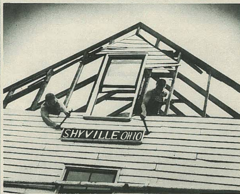
An atomic bomb didn't exactly create the above scene but as a result of the new atomic age the last of the little community of Shyville, Ohio is being removed to make way for the Portsmouth Area plant. Pictured removing the old post office name sign are workmen John Collinsworth (left) and D. C. McCorkle. The old post office is one of the last buildings being torn down within the project area.
