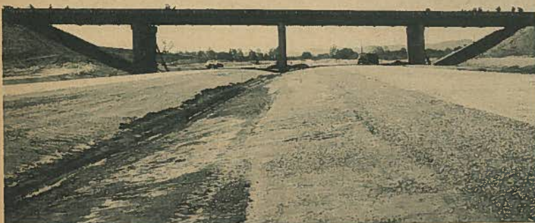
Rapidly nearing completion is the overhead crossing (partially shown above) which will serve as the principal access entrance from new U. S. Route 23 into the jobsite. Highway officials said the new overhead and the section of four-lane roadway between Wakefield and Piketon is slated to be opened to traffic on or before July 1. (See story on page 1).
