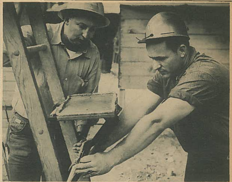
Shown checking a portable ladder platform being used by Reynolds-Newbery electricians in the construction area, is Electrician G. M. Wolfe (left) and Welder F. Shinn. The devices which are being made on the job enable electricians to work for longer periods of time and with much more ease on ladders. The stands which have been praised by the PKS Safety Department, will fit on any standard ladder rung.
