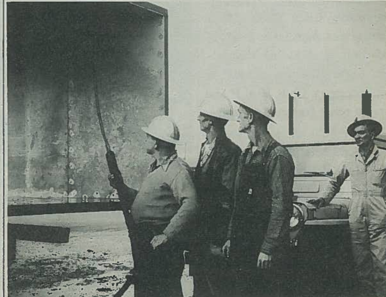
Steam cleaning of all sheet metal going to buildings is the job assigned to "Shorty" Hooper at the storage yard. Assisting him are sheet metal worker C. A. Spicer and operating engineer J. C. Botkins. Teamster R. George watches on as he waits to pull his farm wagon of metal to be cleaned.
