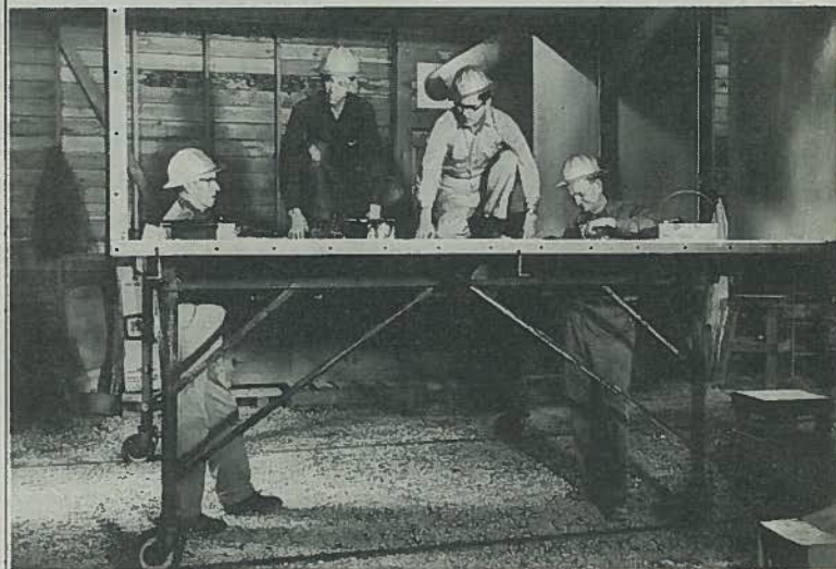
Shown working in the assembly shop about to join together duct are sheetmetal workers (left to right) B. D. Parsons, E. S. Gresham, F. F. O'Connell, and D. A. Silliman. This phase of operation follows the delivery of materials from the storage yard.
